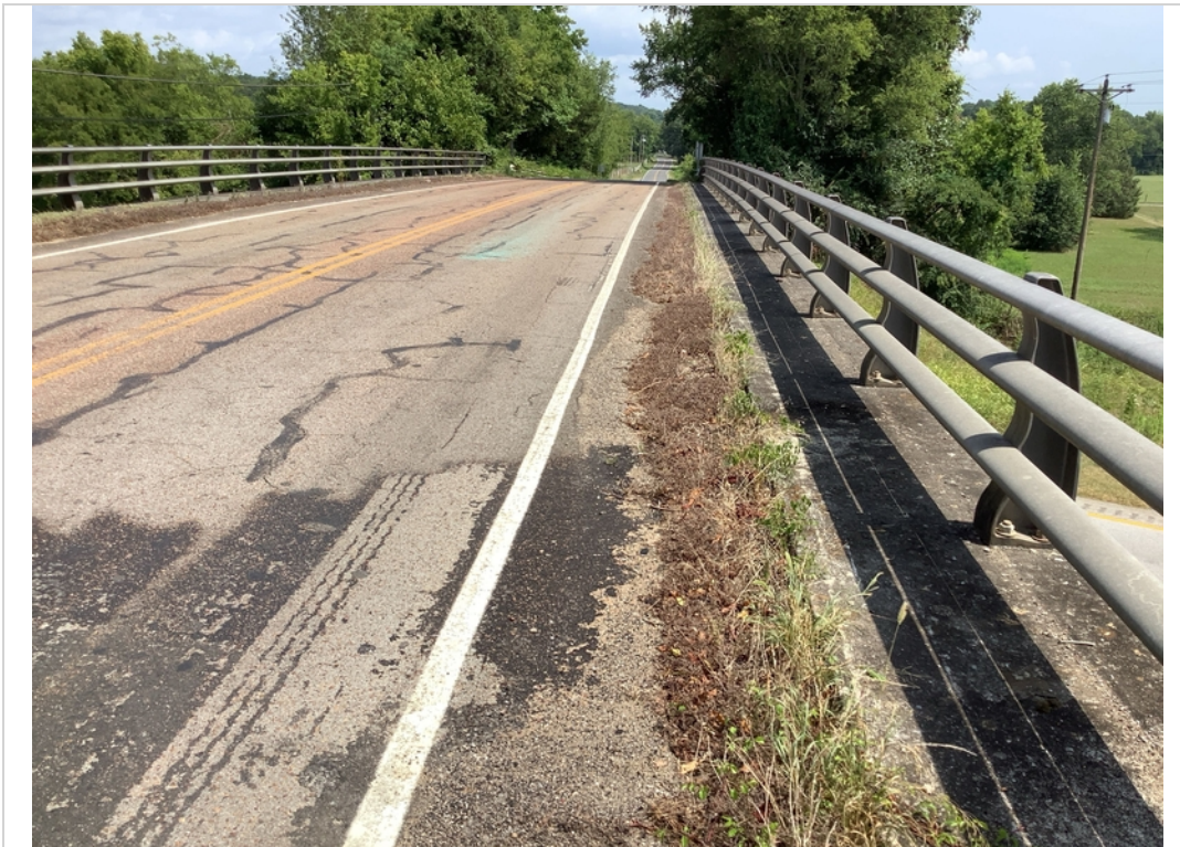
Debris on top of deck
