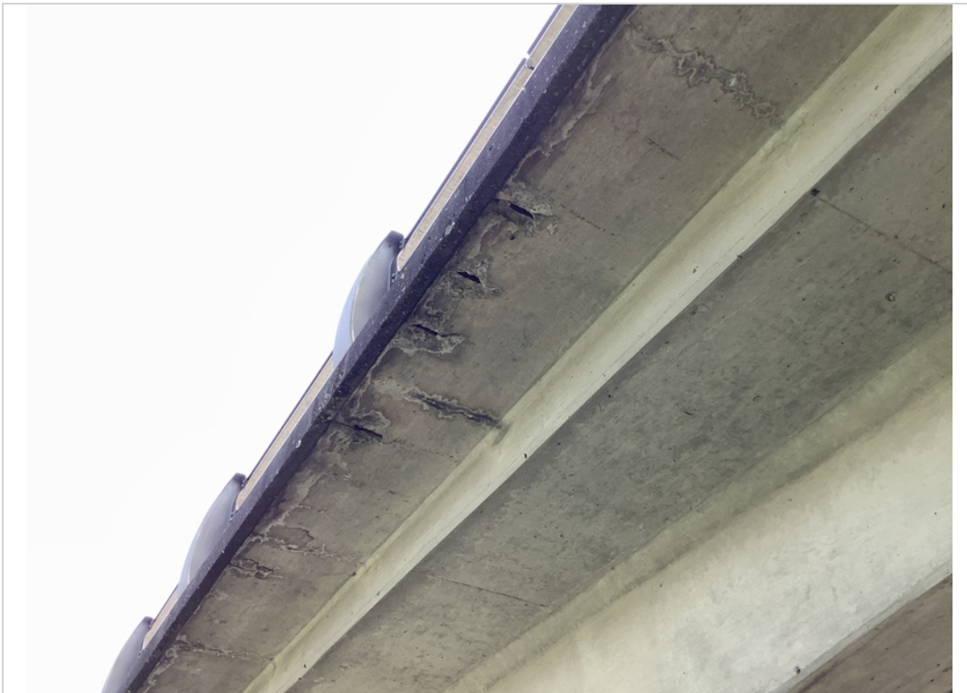
Typical spall with exposed rebar
